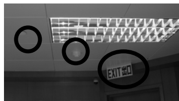
(b) Fire detector, concealed sprinkler and emergency exit sign
