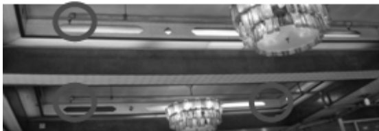
FIGURE 3. Sprinkler in the restaurant in EB2
