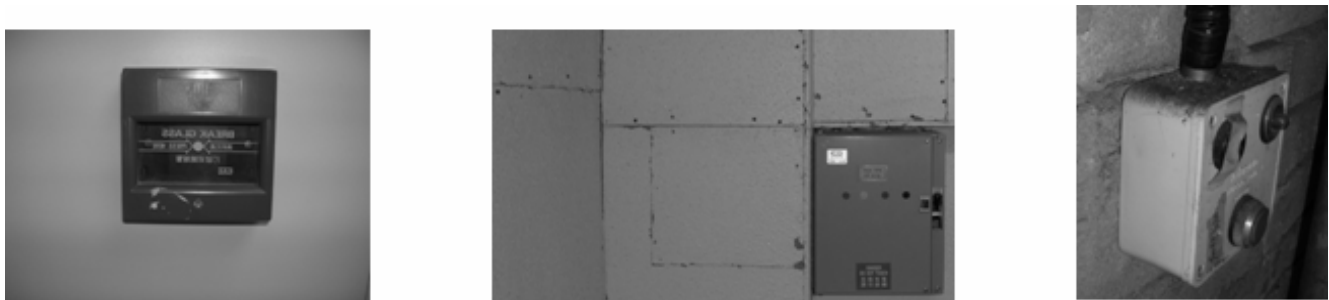
(e) Manual alarm call point (f) Essential power switch (g) Deteriorated sprinkler pump manual starter
